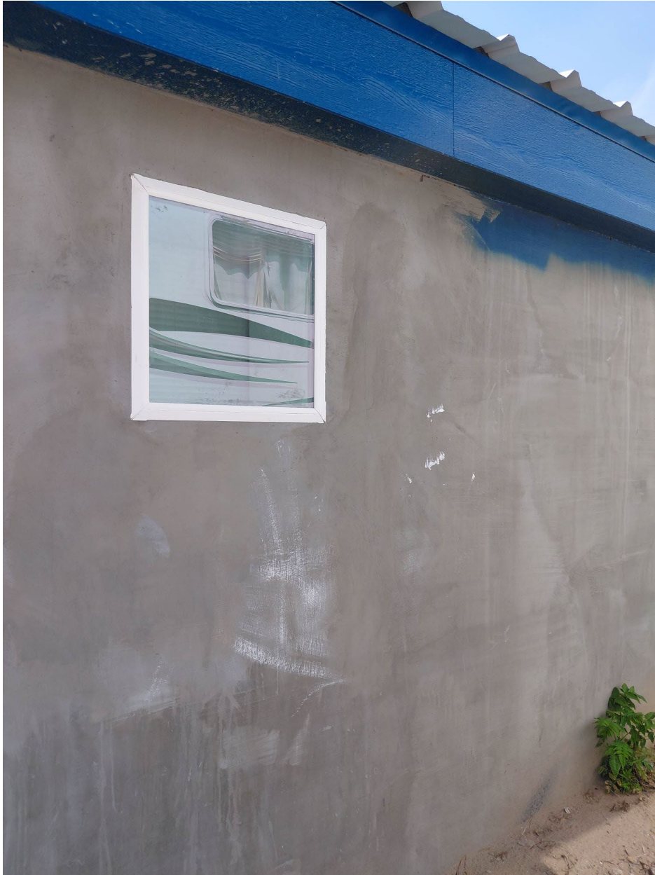
Figure 11: Former location of steel casement window with transom, now a fixed inoperable window.
