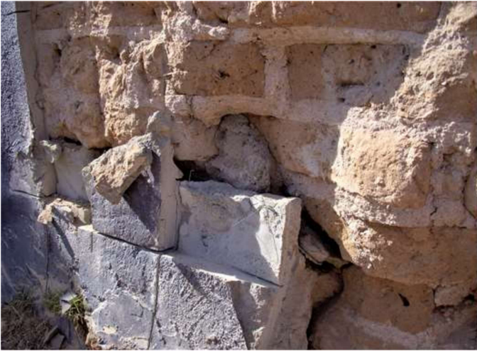
Figure 22: Basal wall deterioration at the Apse. (Courtesy of Faith Hutson)
