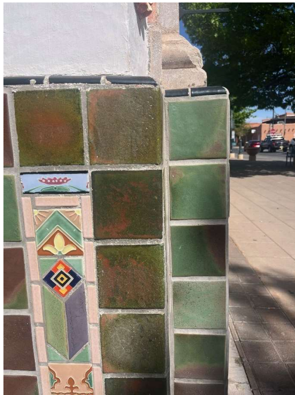
Figure 9: Original and replicated tiles on the theater exterior.
