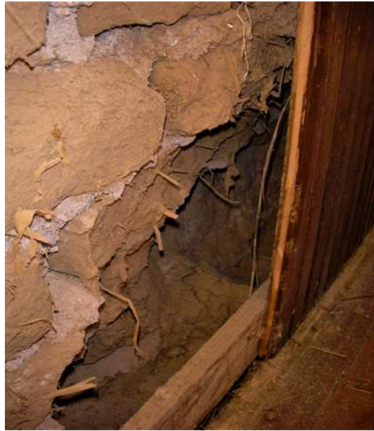
Figure 23: Basal wall deterioration inside. (Courtesy of Faith Hutson).
