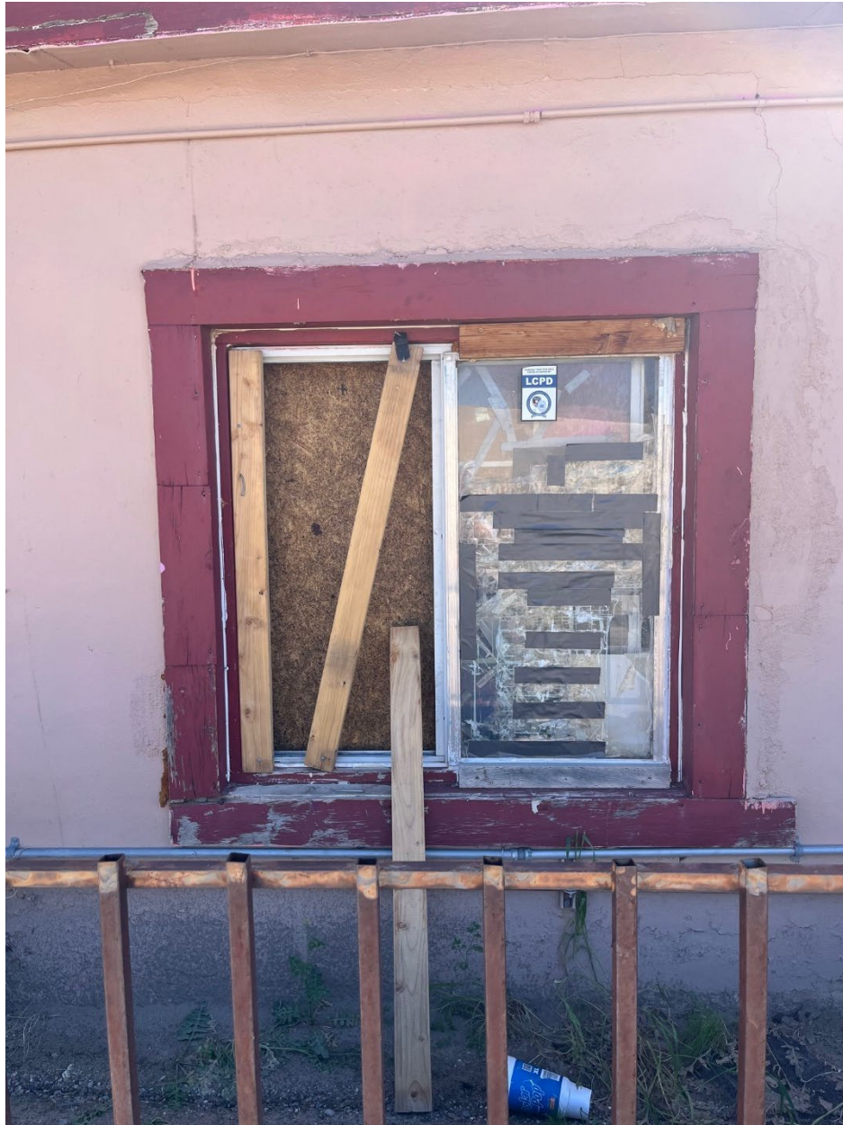
Figure 6: Window on the house facing Lucero Street.
