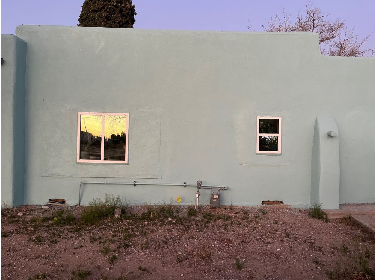
Figure 11: Example of improperly-installed replacement vinyl window, with the original cavity poorly filled-in.
