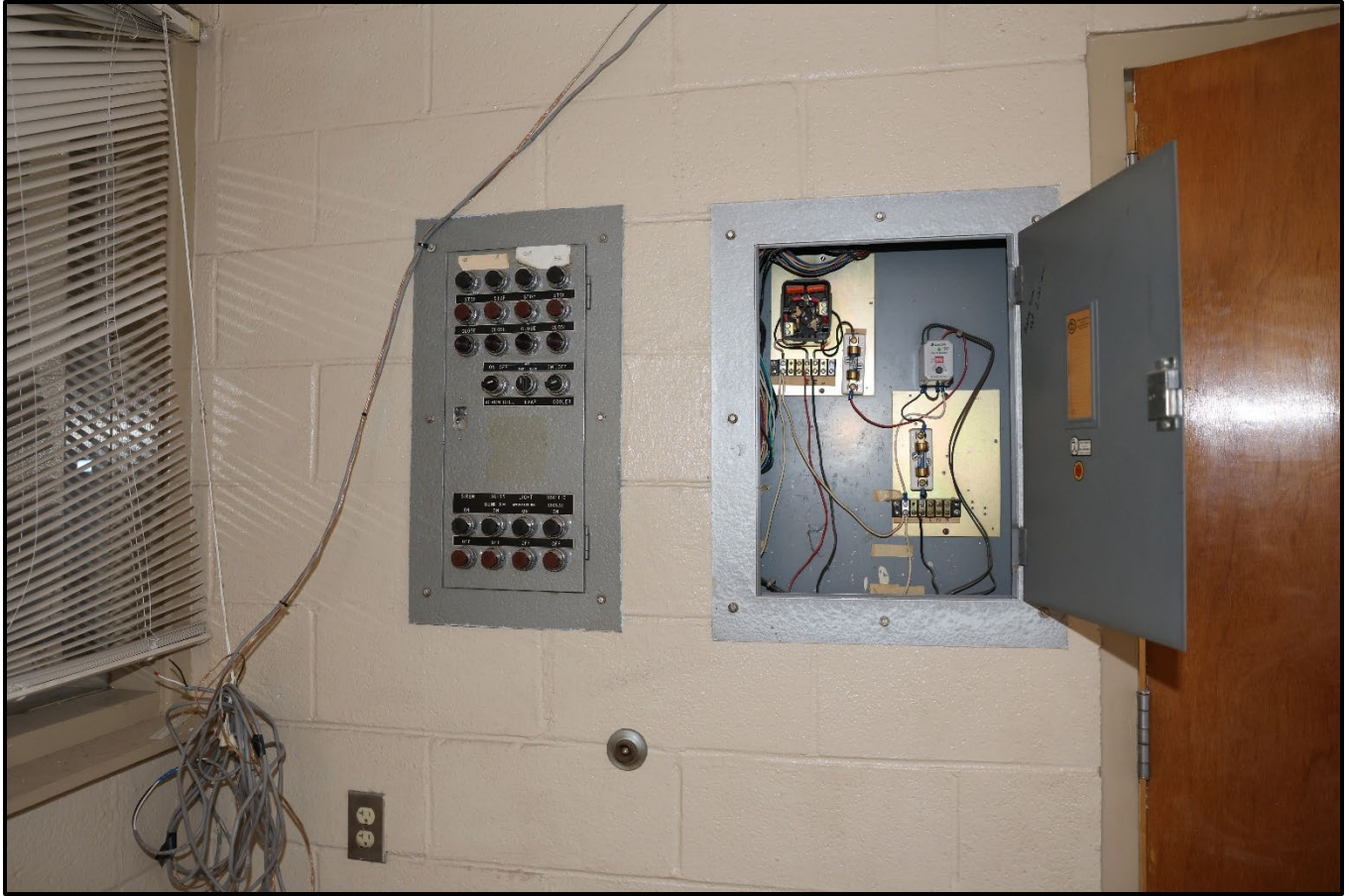
Figure 38: Photo of fire alarm control panel and switch board in the duty room.
