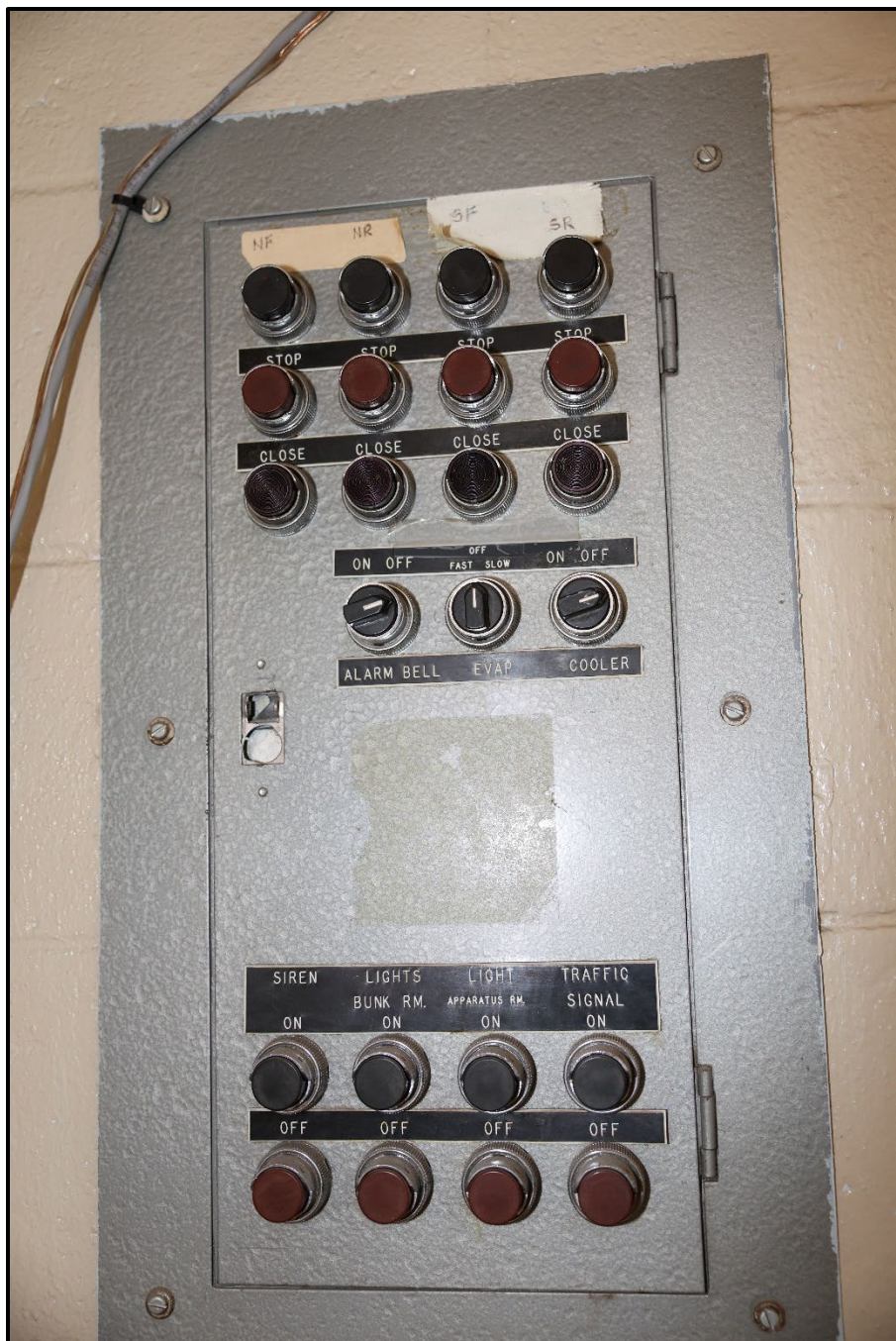
Figure 39: Detail of the fire alarm control panel.
