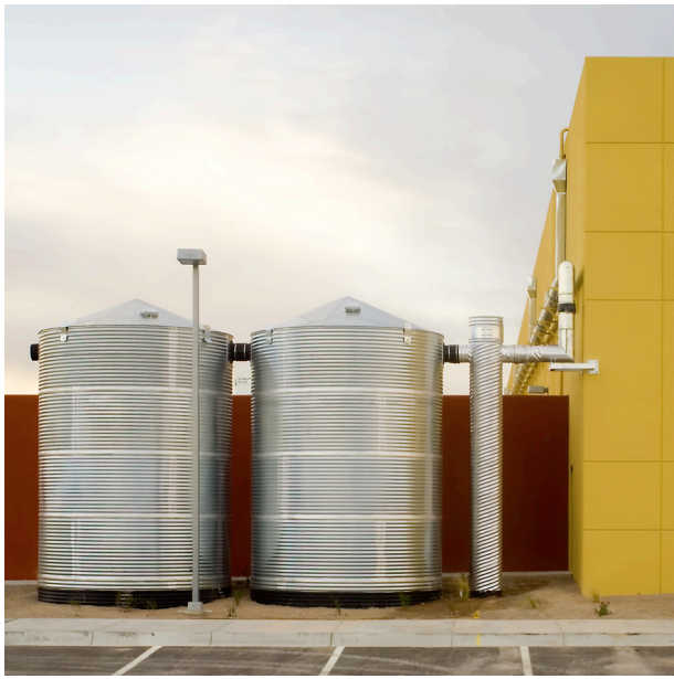
Cisterns to capture runoff from building roofs
