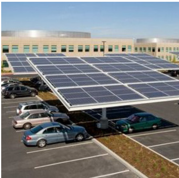
Energy production through Solar covered parking lots
