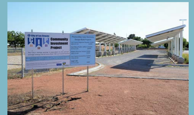
The City has invested in solar panels at many municipal facilities to generate energy (below).
