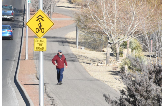
The pavement surface on the Triviz Multi-use Trail is in good condition.
