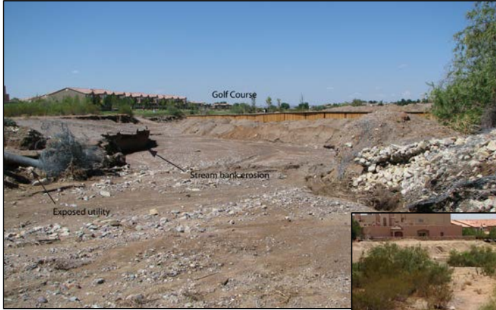
Flooding near the Sonoma Ranch Golf Course inspired a simple and inexpensive naturalistic erosion measure (below) which preserves natural vegetation and blends in with the surrounding terrain. Both photos: CLC Public Works Dept.
