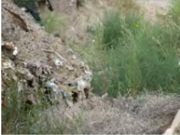
Photo #1 Eroded area on north side of tract 9AR2, exposing debris.
