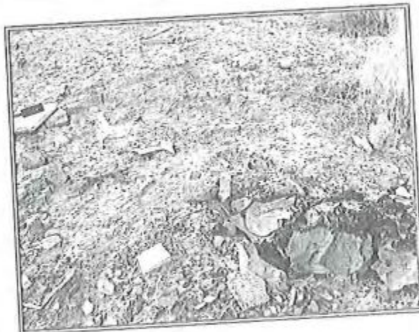
View of suspect ACM
