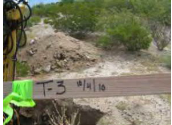
Photo #2 Test pit 3, debris.
