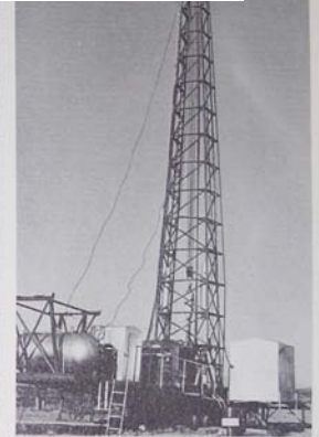
MORE WATER—New wells drilled in 1965 mean adequate water for a growing city now and in years to come.
